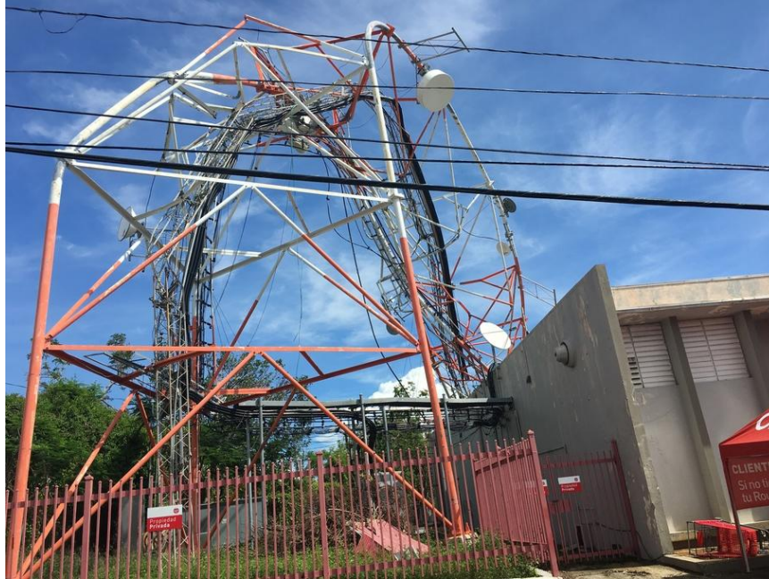
Figure 1.2: Devastation in Puerto Rico from Hurricane Maria in 2017 included most of the communication infrastructure on the island. FEMA/Richard Cardona https://www.fema.gov/media-library/assets/images/151854#details
